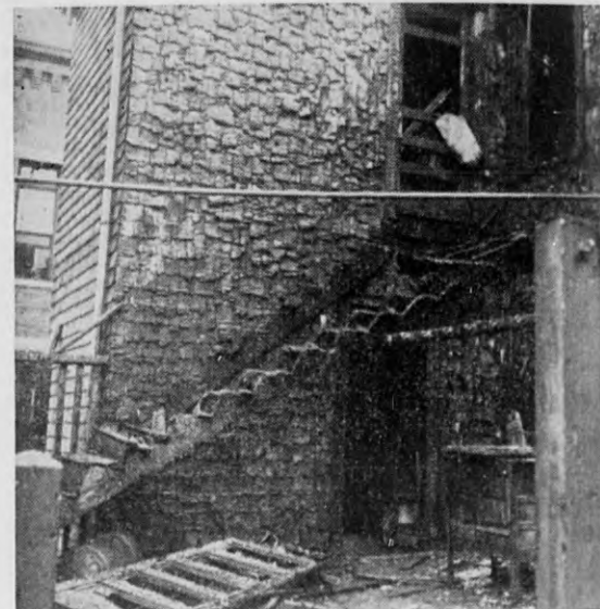
How would you like to go up those stairs? This is what was left of the rear of the Elm block Friday morning.
