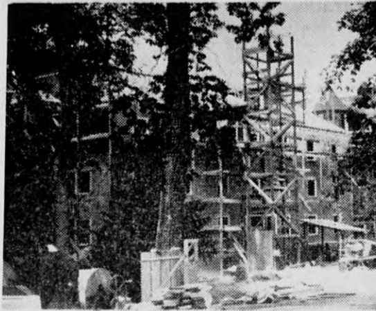
Work is rapidly progressing on Abbot Academy's new dormitory, the first physical development arising out of the Twentieth Century Fund.
