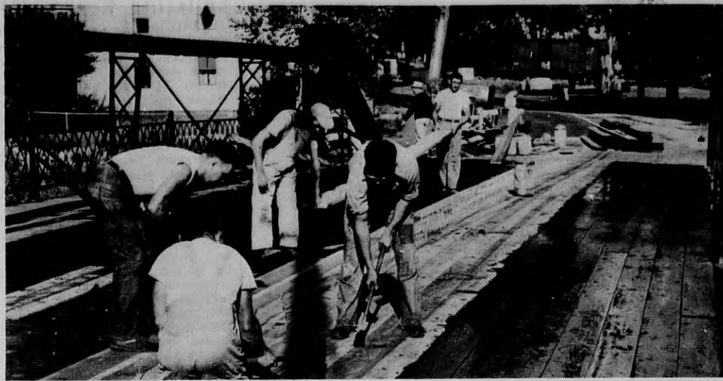
Putting a new flooring on the bridge over the Shawsheen river at Andover street in Ballardvale, workmen for the board of public works are shown putting the top layer in place, part of which has already been treated with a preservative. The bridge has been entirely retimbered after the finding of so much decayed woodwork under the flooring. (Look Photo)
