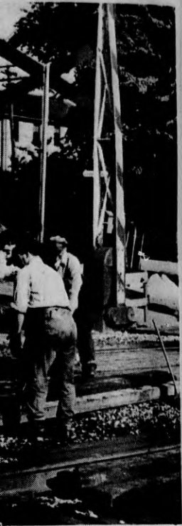
place the upright in the sewer type gates and flash- (Look Photo)
