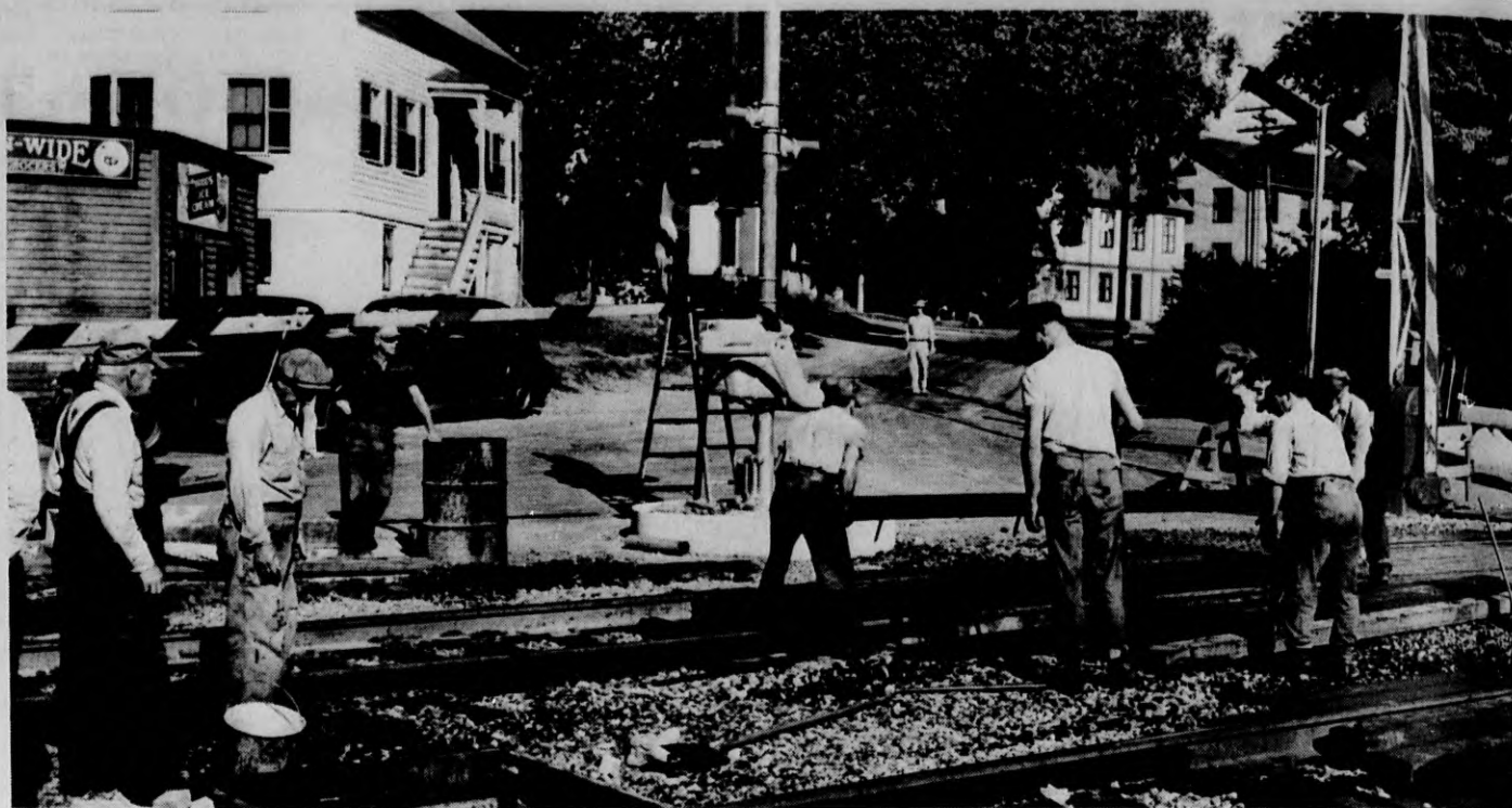
In connection with the work of installing new automatic gates at the Andover street crossing in Ballardvale, workmen for the railroad have raised the tracks here and are putting in new planking for the
