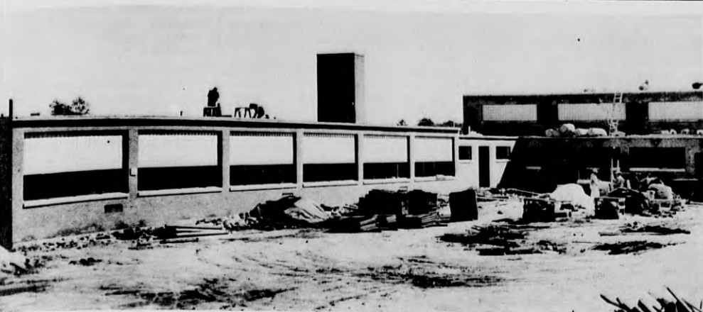
The new West Andover grade school nearing completion to take care of the growing needs of the younger children of that district. The one-story building will have six rooms with an auditorium, cafeteria and offices. (Look Photo)
