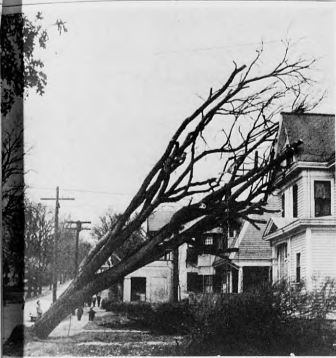
Large elm tree that was blown over onto house at 121 Main street during the wild northeast storm that struck the town last Saturday with pelting rain. Upper windows were smashed and part of the roof damaged. The tree department has removed the tree. (Look Photo)
