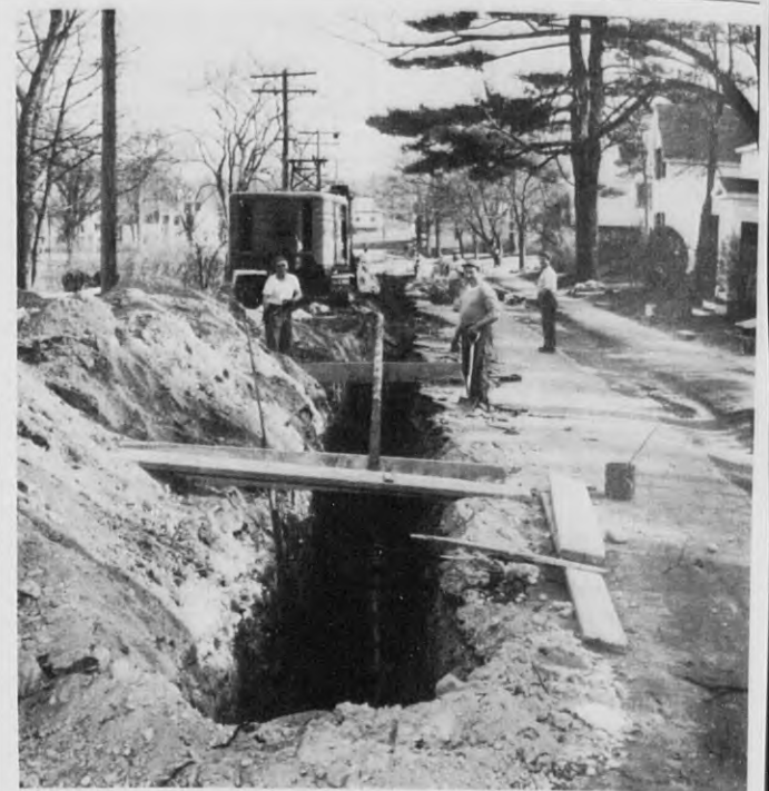
Photo showing one of the phases of the new Ballardvale sewerage system now being installed. This trench on Andover street is one of several that were opened in streets about the Vale center for pipes that will run under the Shawsheen river and the railroad tracks to connect with the treatment plant near Dale street. (Look Photo)
