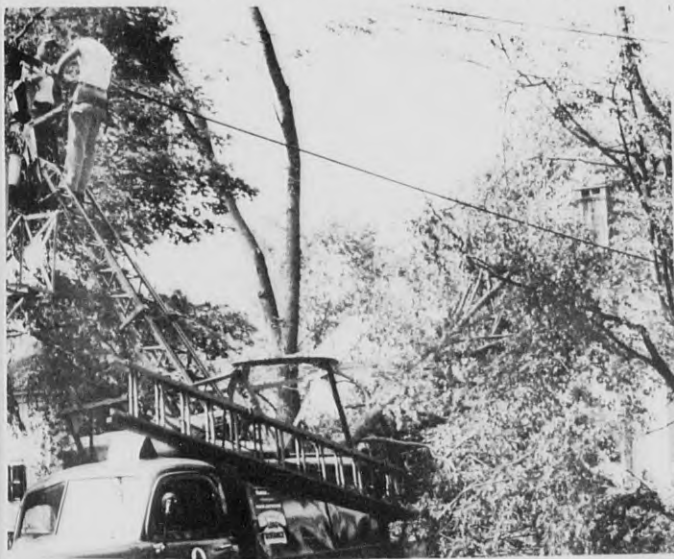
Familiar sights around town since the hurricane are the repair crews of the N. E. Tel. & Tel. Co., similar to this cable-splicing team at work on Summer street. (Look Photo)
