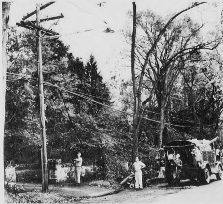
Repair crews from New York and Vermont are shown here replacing damaged telephone cables and wires that were felled on Central street near St. Augustine's school at the height of the recent hurricane. (Look Photo)
