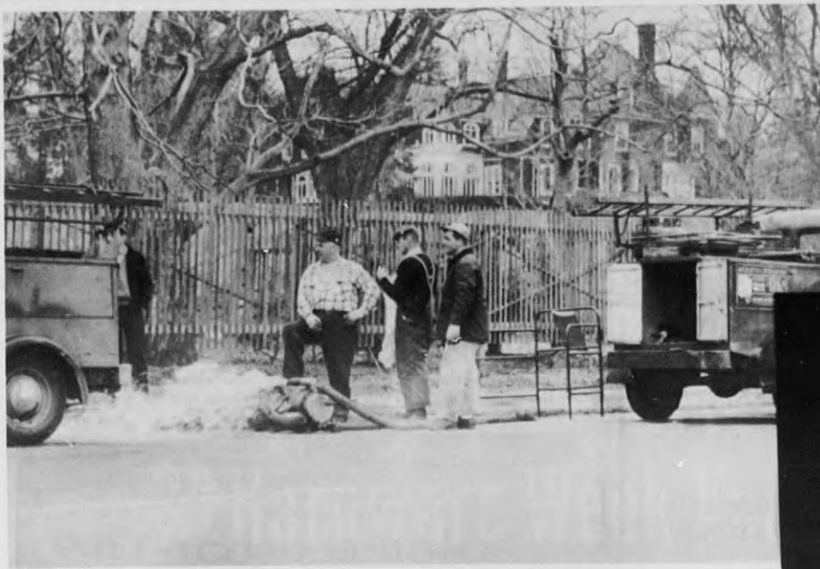
The Lawrence Electric company had a busy time here last weekend, as the heavy rain caused underground wires to short out. Many homes were left without power for several hours. This crew is working on Main st. in front of the Wood estate.
