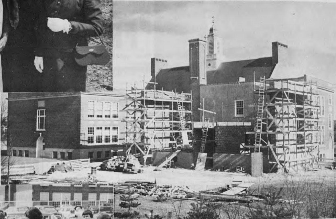
Construction of the Shawsheen school addition is coming right along, as this Tuesday afternoon photo indicates. (Leone)
