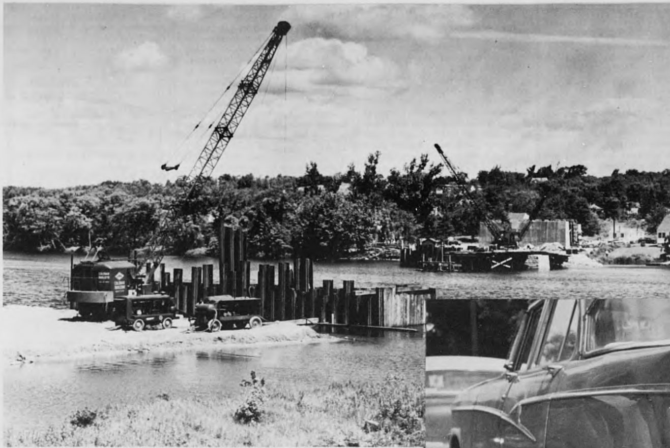
The sub-structure of the Route 28 bridge across the Merrimack river is progressing rapidly. At left is the work on the Andover side of the river, while across the stream is the more-nearly finished Methuen portion of the structure. (Leone)
