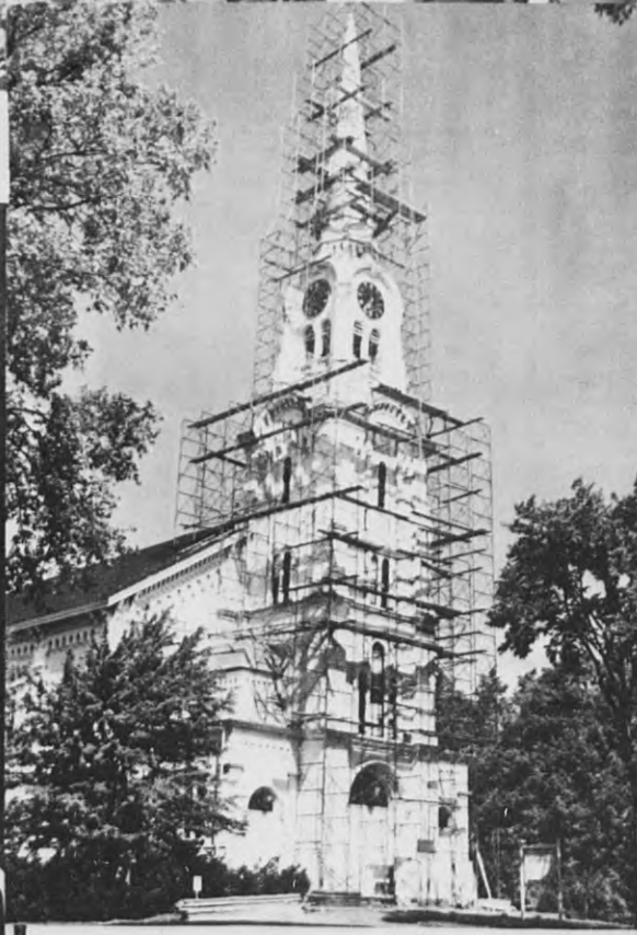
Work on the South church steeple is progressing, with most onlookers wondering who wants to climb that high to do a day's work. (Leone)
