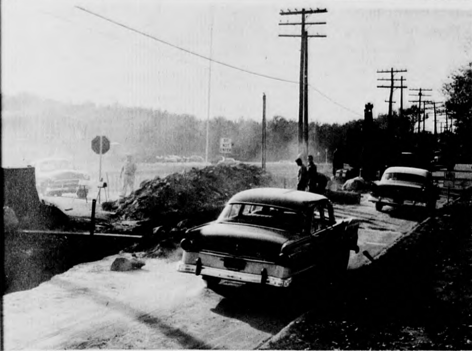
TRAFFIC IS IMPEDED - Shawsheen rd. reconstruction has slowed traffic down to a creep, as town crews and contractors work on lowering water and drainage pipes. The actual road reconstruction also is progressing satisfactorily, according to Water Dept. Supt. Donald Bassett. (Leone)
