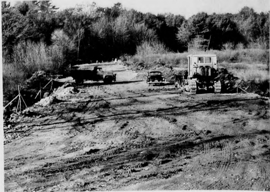
WIDENING BALLARDVALE RD. - Town crews have been busy the past 10 days dumping fill and levelling it on Ballardvale rd., to widen the street. Highway Supt. Stanley Chlebowski said the work will continue for some time.
