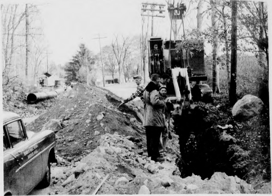
WATER MAIN CONSTRUCTION - Porter rd. is currently being torn up to make way for the 16-inch water main that will carry 500,000 gallons of water daily from the Ballardvale test well. Water Department Supt. Donald Bassett, foreground, has said the work is going according to schedule. The DiMartino Construction Co. is doing the work. (Leone)
