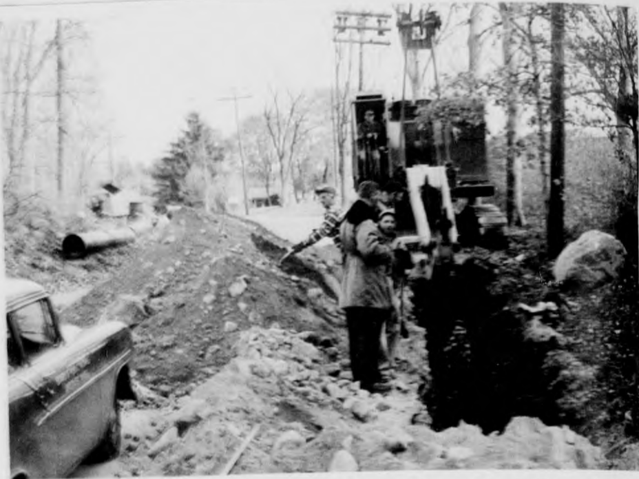
WATER MAIN CONSTRUCTION - Porter rd. is currently being torn up to make way for the 16-inch water main that will carry 500,000 gallons of water daily from the Ballardvale test well. Water Department Supt. Donald Bassett, foreground, has said the work is going according to schedule. The DiMartino Construction Co. is doing the work. (Leone)
