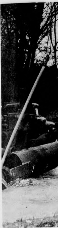
BALLARDVALE TERRACE permanent well in Ball... They should be moving... Water Dept. Supt. Don...
