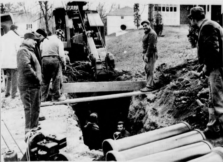
IT'S A DEEP ONE - The Castle Heights-Juliette st. sewer goes quite deep through some of the back yards, as workmen rush to get as much done as possible before bad weather. The BPW has authorized Supt. Donald Bassett to halt the construction whenever he thinks it necessary because of frost and general conditions. (Leone)
