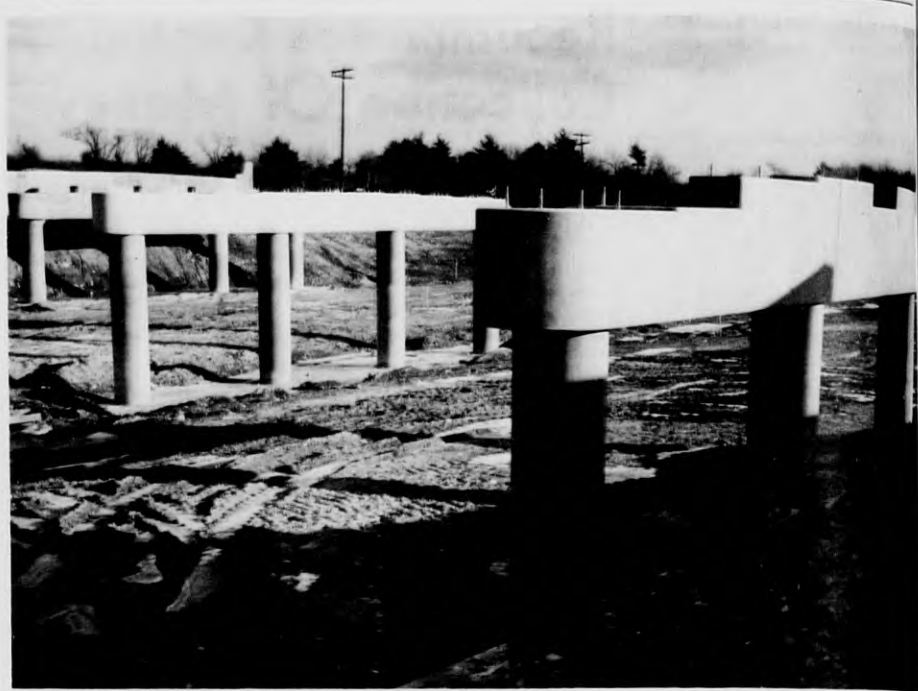
ROUTE 28 - These over-pass foundations are in place for Route 28, as it goes over Shawshen rd. Work has been continuing on the Andover sections of the road at a rapid rate throughout the fall and winter. (Leone)
