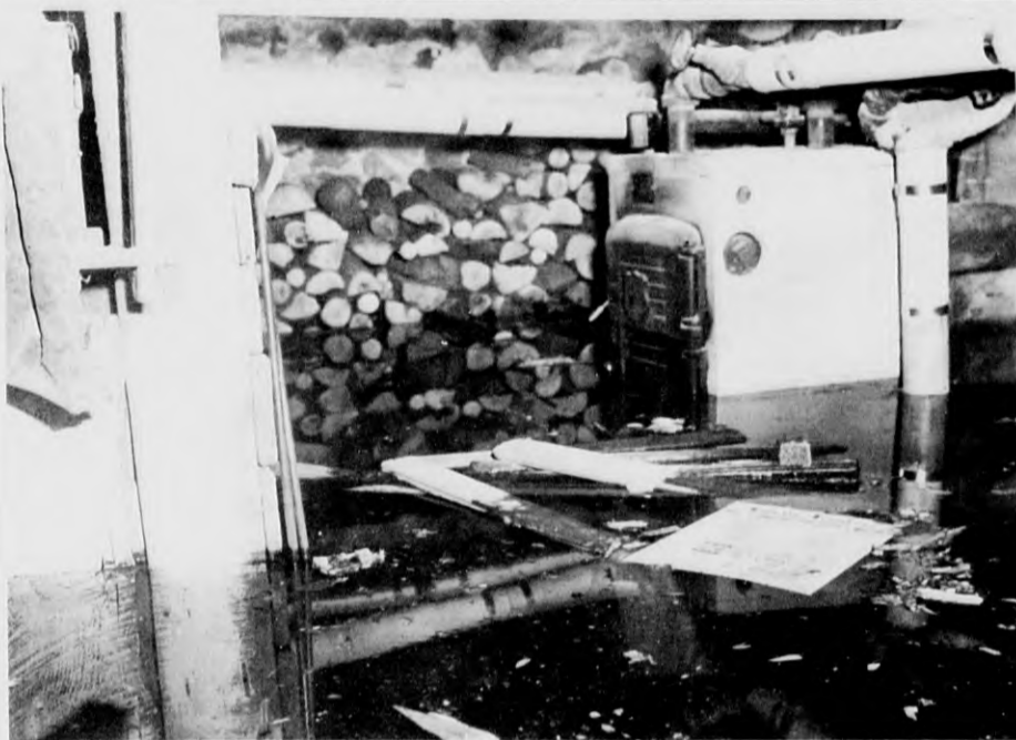
VICTIMS OF THE STORM - The Fred Oldroyd home on Center st., Ballardvale, was heatless, following the weekend downpour. Fred measured four and a half feet of water in the cellar. His new furnace is a complete loss. (Leone)
