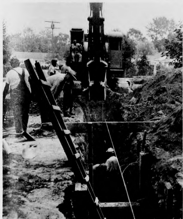
DEEP - AND HOT! This is the Shawsheen Hylands sewer, just as it enters Marwood dr., off Lowell st. Workmen handling the air hammer in the trench had a mighty hot job on a muggy Monday afternoon. The Susi and DeSantis firm is handling the project for the town.
