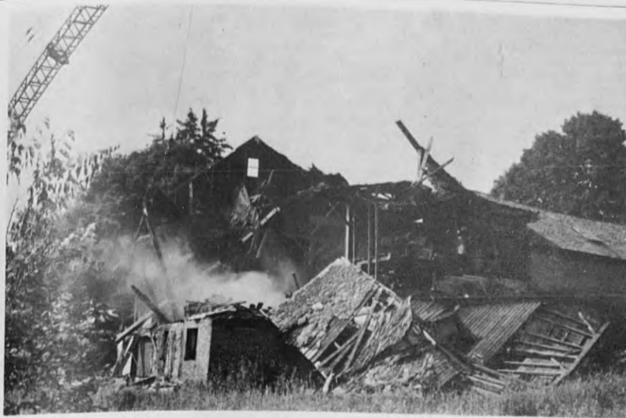
LANDMARK DISAPPEARS - A giant crane swiftly tore down one of the town's old landmarks last week. The barn shown in a partial state of wreckage here goes back about 135 years, and belonged to Mrs. George Abbot on Upland rd. When the barn was built, the street was known as Summer st., with the name changing when the present Summer st. was extended to Highland rd. (Cole)
