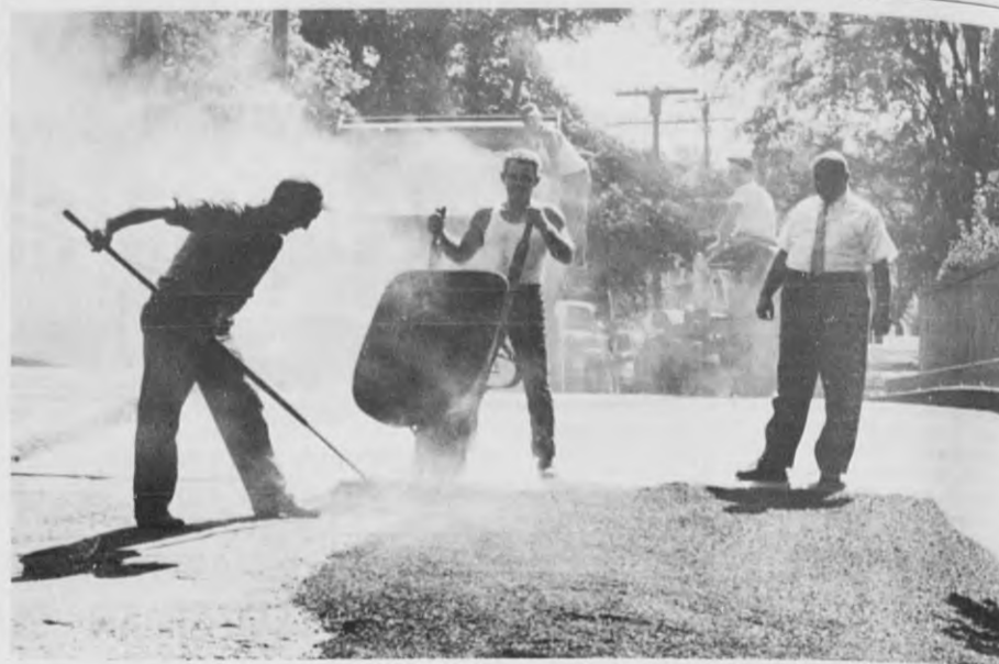
SMOOTH RIDES for motorists resulted from the resurfacing of several streets in the town during the past two weeks. Shown at work on Harding street are, left to right, John Lynch, James Buss and Highway Superintendent Stanley Chlebowski. In the background on the truck are Dudley Young and William Floyd. (Leone)
