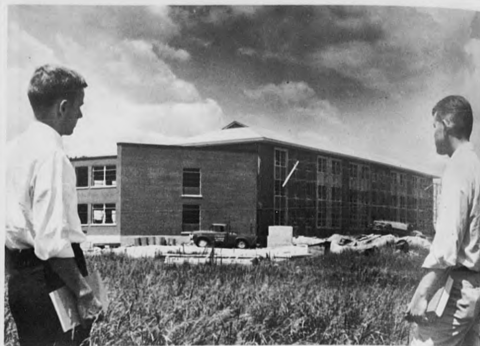
GIRLS DORMITORY at Merrimack College is nearing completion. Shown looking at the new structure are two summer students, Robert Walsh, left, and James Dorsey, both of Andover. (Leone)
