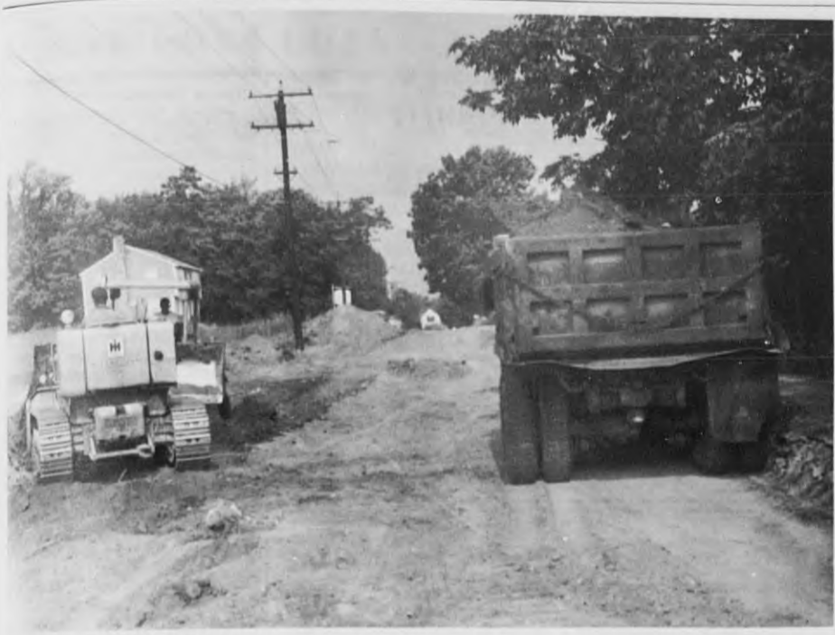
DASCOMB RD. BOTTLENECK - Chapter 90 reconstruction of Dascomb rd. has produced one of the town's worst traffic conditions. While work is in progress daytimes, traffic has to thread its way between the working machines, and around exposed manhole covers. At night, cars have to creep through the area, winding their way around the manholes. The road is being widened and resurfaced under the Chapter 90 allocation. (Staff Photo)
