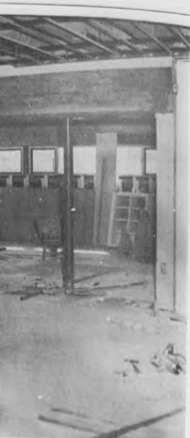
Hall Library has taken shape. Believe the job may be completed by the end of the year, facing the portion of the building. (Staff Photo)
