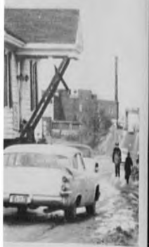
on of house moving. This on the last lot before the on st., as workam lifted e of the street. (Staff photo)
