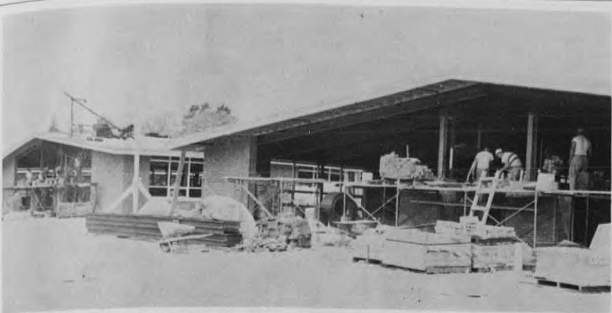
READY BY SEPTEMBER - These are two of the three wings of the elementary school on Lovejoy rd., which will begin serving pupils this September. The portion of the right-hand wing in the foreground is the kindergarten area. Three wings extend back from an office and service area across the end. (Staff Photo)
