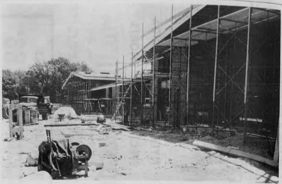
HURRYING CONSTRUCTION - The new elementary school on Lovejoy rd. has been a bedlam of activity, as work is rushed to have the classrooms ready for occupancy when school opens in September. This is a view of the administration and service areas. At far left will be the administration office; the cafeteria will be housed in the central area, and at right is the gymnasium, with the staging still in place. Clerk of the Works Edward P. Hall said progress indicates the school will be ready for classes in September, even if the service areas are not quite finished. (Staff Photo)
