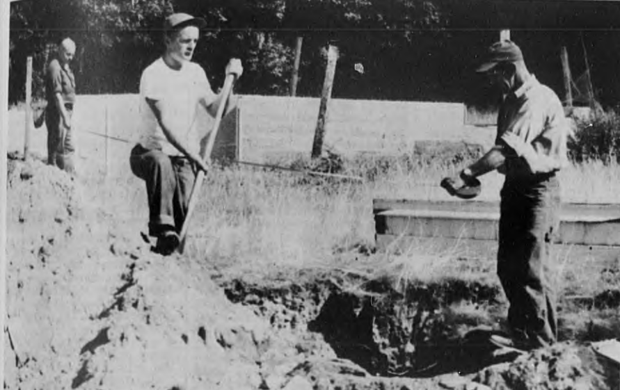
SHUTTING OFF SERVICES to abandoned homes on Cornell rd. to make way for Route 495 is task now being carried out by the board of public works. Here, from left to right, Francis McCurdy, John Campbell and Foreman David Thomson, are shown as they excavate to the junction of the service with the main where the shut off is made. All of the homes on the right side of the street are being moved. The town employees also recover, whenever possible, the water meters from the buildings. The service pipe, from the main to the home, is left in the ground. (Cole)
