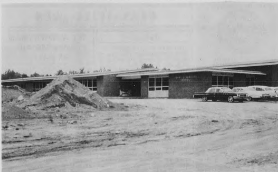
ALL BUT COMPLETED - The Henry C. Sanborn school on Lovejoy rd. is nearly completed, and will be ready for classroom occupancy when school opens. One of the remaining tasks is grading and hot topping the area - the big pile of fill at left is only one of many that must be moved before the external work can be finished. This has been said to be the only remaining possibility for delay in opening the school, but the contractor believes he will have the work well underway, so that school can open as scheduled. (Staff Photo)
