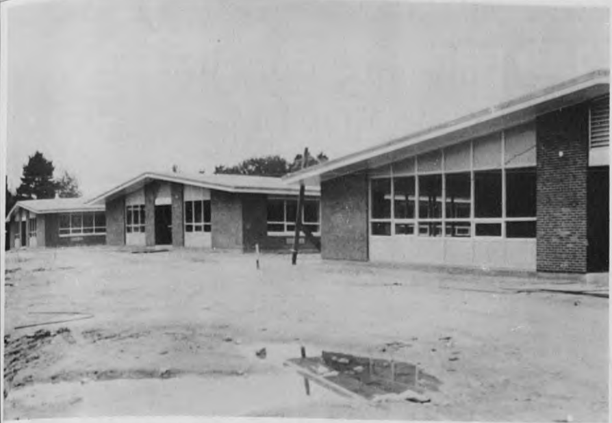
THREE WINGS of the new Henry C. Sanborn school on Lovejoy rd. are shown in this photo. At right is the kindergarten wing, others will house other grades. Nearly all of the interior work is finished, and equipment is being installed. (Staff Photo)
