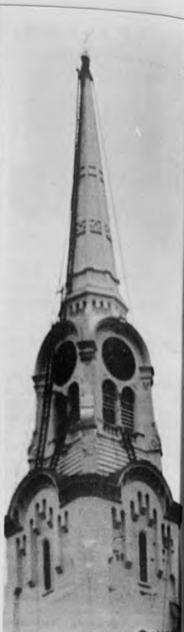
ATOP SPIRE - It's a risky job, at best, in our view, but the workman at the very tip of the South Church steeple Monday morning seemed to be working away without concern. Not our idea of pleasant working conditions - but everyone to his own.
