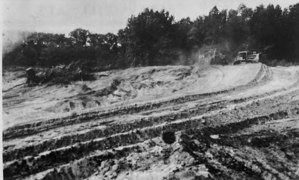
FINALLY UNDERWAY - Earth, trees and scrub growth gave way before the contractor's heavy equipment at the High School recreation site, after a contract was finally awarded for this sub-grading and drainage project. Original bids were tossed out, and second bids called for, in order to come within the town's appropriation of $40,000 for the work. Residents over most of the town have been able to see the tall column of smoke coming from the area, as the contractor burned the trees and brush. (Staff Photo)
