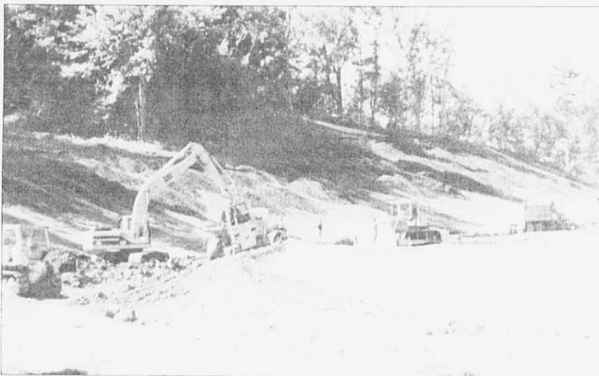
Crews of heavy equipment prepare the entry road to Great Hill prior to paving and landscaping.
