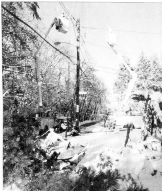
Power was out for nearly 15 hours as a tree fell at the intersection of Highland Avenue and Heather Drive.
