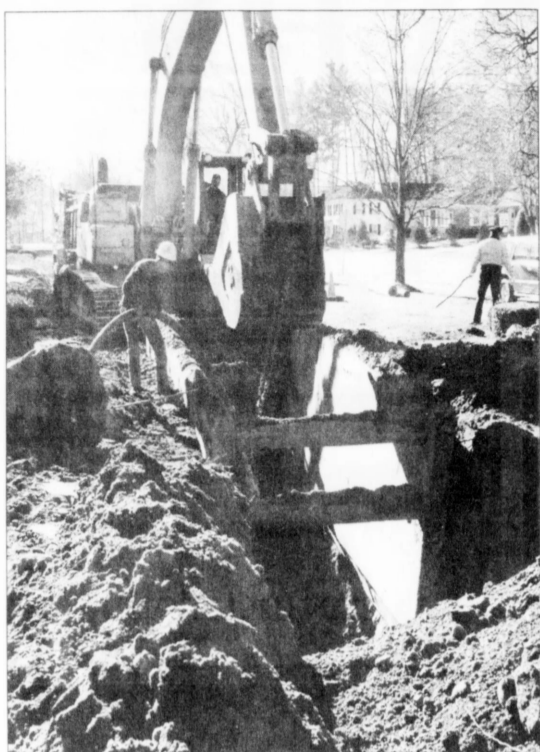
Workers will continue working on Route 28, Andover's Main Street during the next year. The entire sewer expansion won't be complete for nearly three more years.
