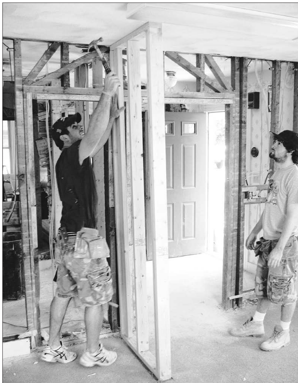
Ben Perkins and Andy Anketell work on restructuring the first floor of 37-39 Pearson St. on June 2, the future temporary home of Andover Youth Services. According to AYS Director Bill Fahey, work on the home will continue this summer in coordination with one of the department's community service programs. Carpentry will give way to sanding, painting and wallpapering in preparation of an Oct. 1 move-in date, he said. "We're excited about the potential it gives us," said Fahey of the former two-family home. Fahey said AYS staff members have received an outpouring of support from the community since selectmen voted May 19 to relocate the department to Pearson Street. Town Meeting authorized the purchase of the home in 2007 to expand the town yard.
