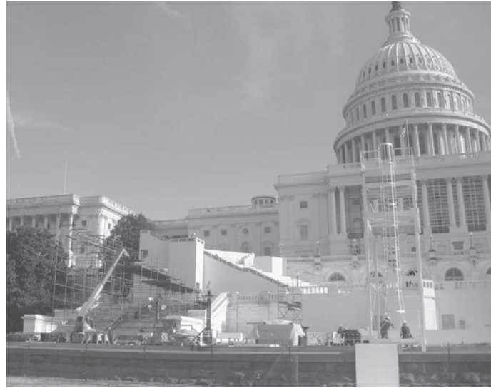
A stage platform has been built on the west side of the US Capitol for the inaugural ceremony.
