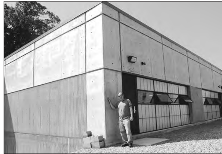
STAFF FILE PHOTO The Robert McQuade Water Treatment Plant on Lowell Street, Route 133, needs roof repairs, according to current DPW Director Jack Petkus.
