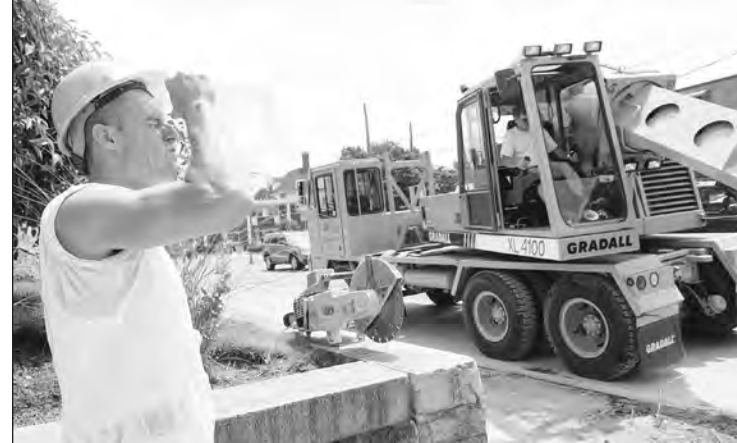
Officials will have a ribbon-cutting at 1 p.m. to celebrate the completion of the more than $2 million Main Street redesign. The ceremony takes place in front of the Town House, 20 Main St. Above, Steve Rice, of S.P. Rice Excavation, poured water onto his face to keep cool last summer while working on the project.
