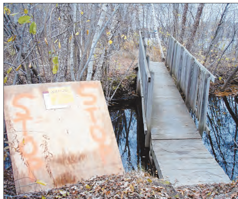
COURTESY PHOTO Andover's Conservation Commission will take down this bridge, which connects a hiking trail over a section of the Merrimack River, on Nov. 14. Members believe the bridge is unsafe and needs to be destroyed before it falls down.
