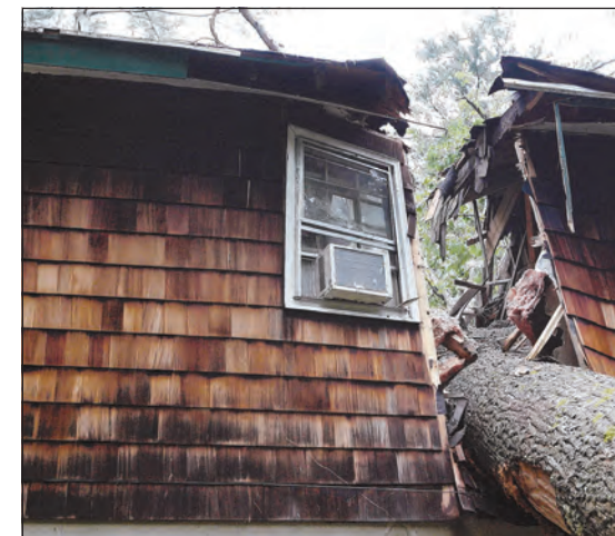
A tree bisects a house in Andover after being uprooted in Saturday's storm.
