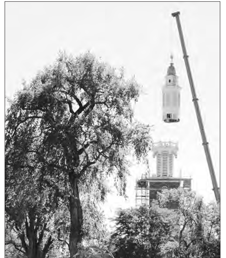
Phillips Academy's bell tower being put into place in September 2005, at the end of its renovation.
