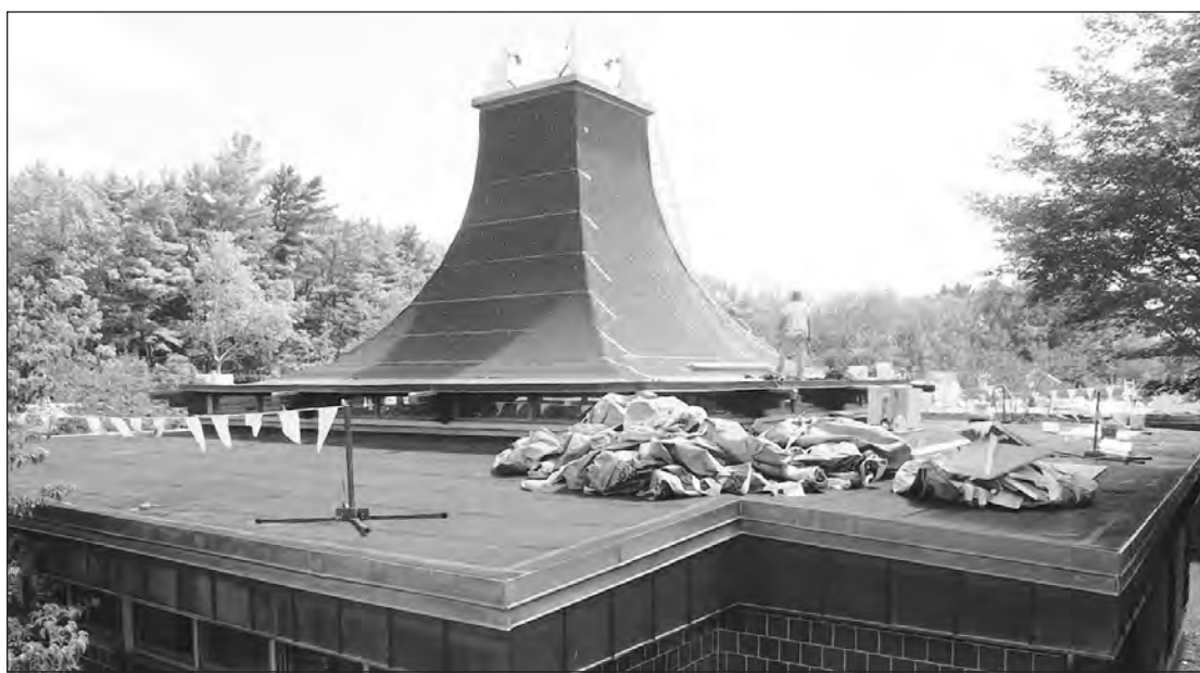
The pagoda in the West Middle School's library is also getting a completely new set of shingles as part of the project.
