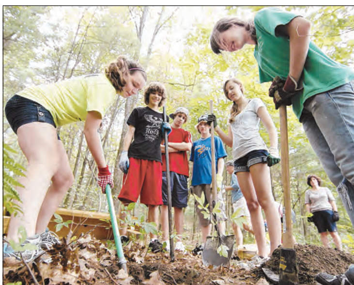
From left, in front, Joanna Olson, Julia Perry, Emily Cardin take turns digging a hole for a bench installation while others helping with the project look on.
