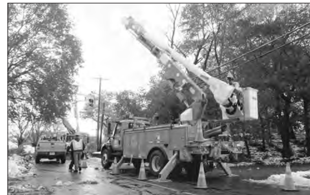
DUSTIN LUCA/Staff Photo Utility crews from Connecticut work to clear tree debris that came down on some utility lines in front of 30 Corbett Street.
