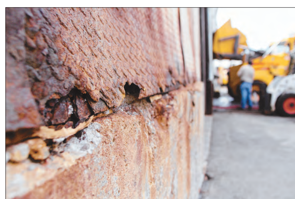
Portions of walls all over Andover's Town Yard are rusting, cracking and peeling away. The facility was built in the 1960s, and they were intended to be used for around 10 years.
