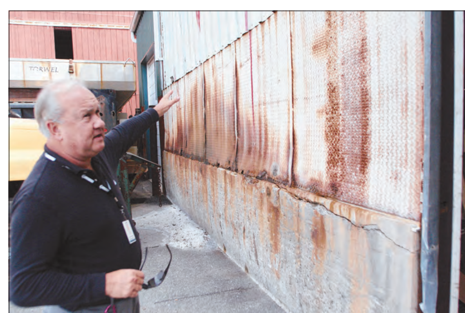
Ihor Raniuk, construction project manager with the town of Andover, shows an area of Town Yard that is rusting and has degraded over time.
