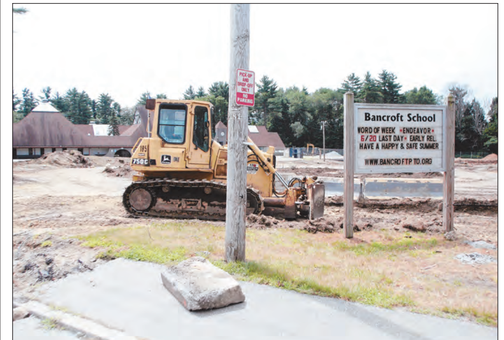
Construction is well under way at Bancroft Elementary School. With groundbreaking about a month away, space once dedicated to playing fields and the school's beloved Dragon's Lair playground has been cleared as part of the project's preparation work.
