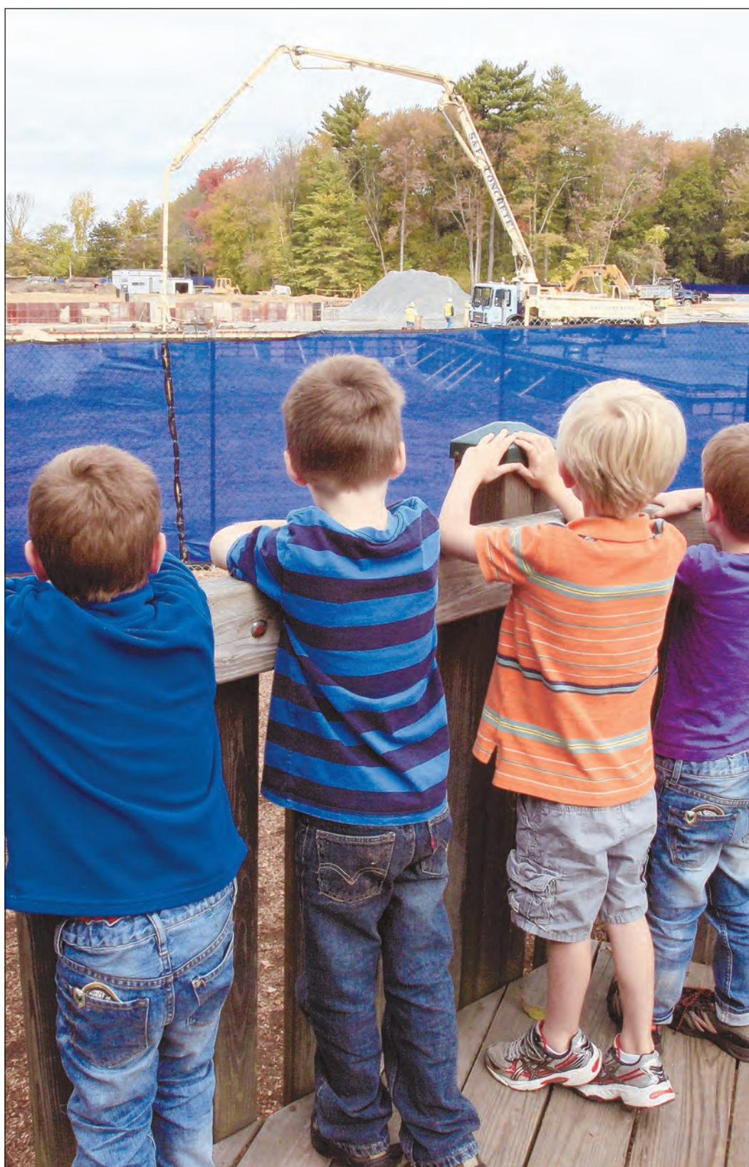
Kindergartners at the Bancroft School grab an elevated view from the top of their playground equipment to watch the new construction during their recess.
