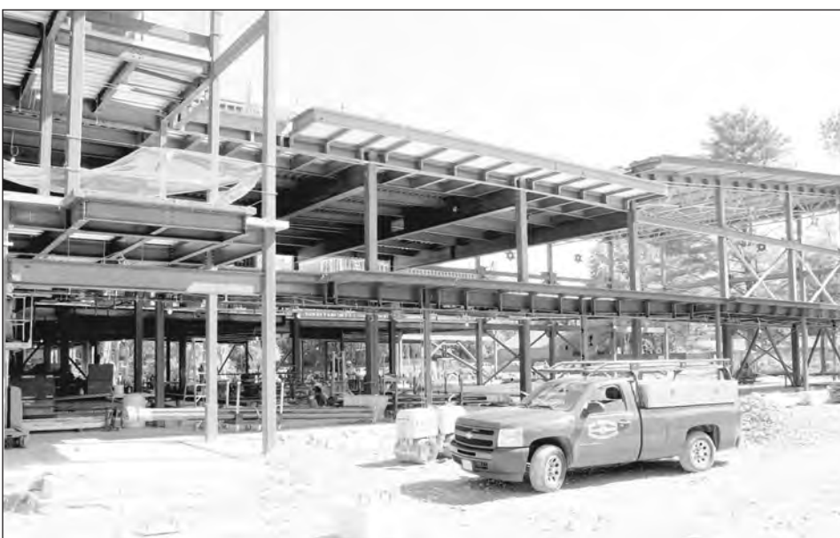
The site of what will eventually be the front doors of the new Bancroft Elementary School, left, is taking shape. Crews will continue putting up the exterior walls and adding the roof this summer.
