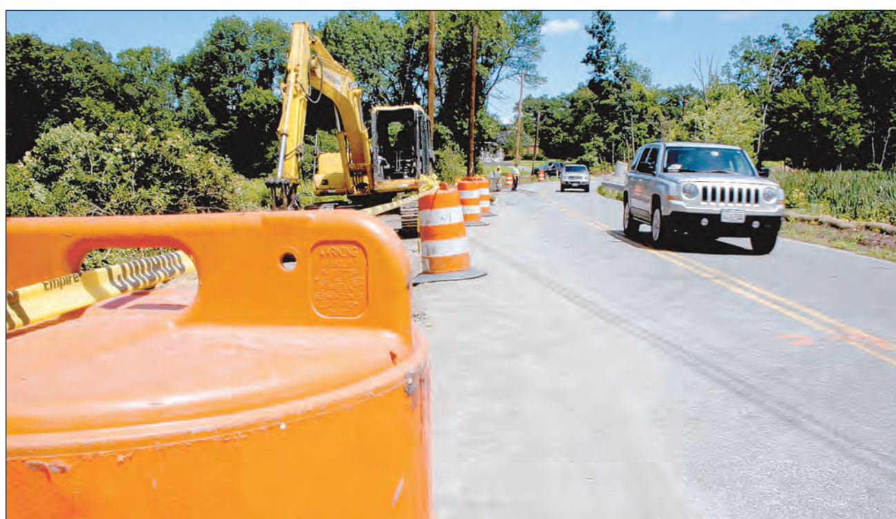
A police officer waves traffic through the construction area on High Plain Road, where work is under way to replace the bridge that cuts through Fish Brook. The road will be completely shut down to traffic next week.
