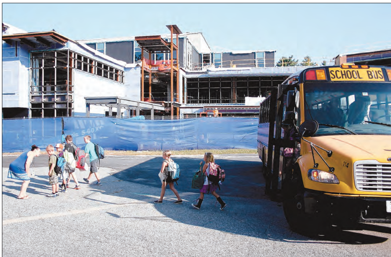
Bancroft Elementary School instructional assistant Cathe Ghandchi welcomes students as they exit the bus on the first day of school last week. A few dozen yards away, construction of the new, three-story Bancroft, which will open next fall, looms over the site.
